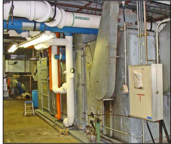
Air Handler AH-2
