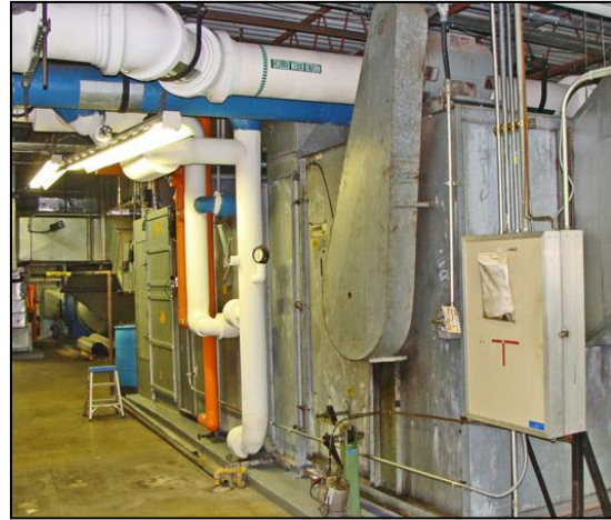
Air Handler AH-2
